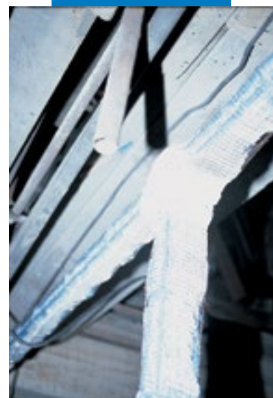
Deteriorated concrete structure
