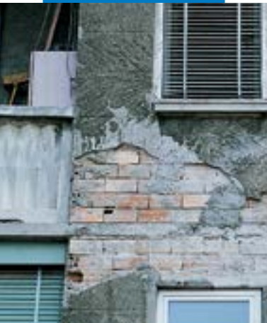
Degraded building façade in need of repair
