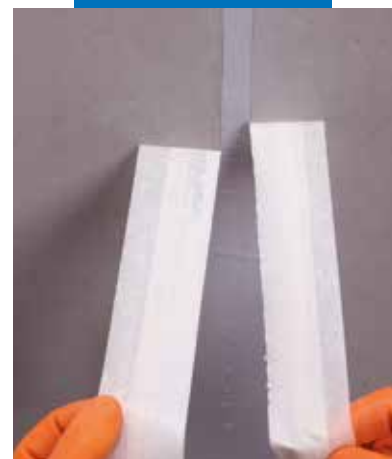
Removal of the masking tape applied around the edges of the joint to avoid rough edges
