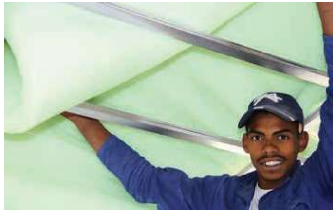
Saftherm polyester blanket insulation cut and snugly placed in the ceiling void between the trusses.
